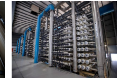
SingSpring Desalination Plant
