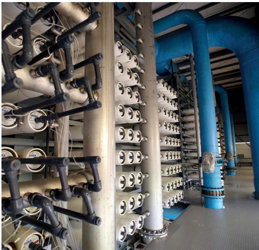
SingSpring (pictured) had used more energy efficient membranes in its water treatment process to reduce energy consumption, lowering Scope 2 emissions by 5% in 2020.
