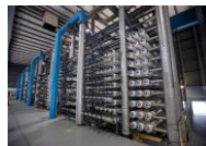
SingSpring Desalination Plant
