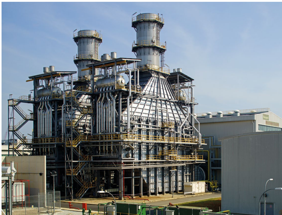
KMC was the first independent power project to enter the Singapore electricity market when the New Energy Market of Singapore was implemented in January 2003.
