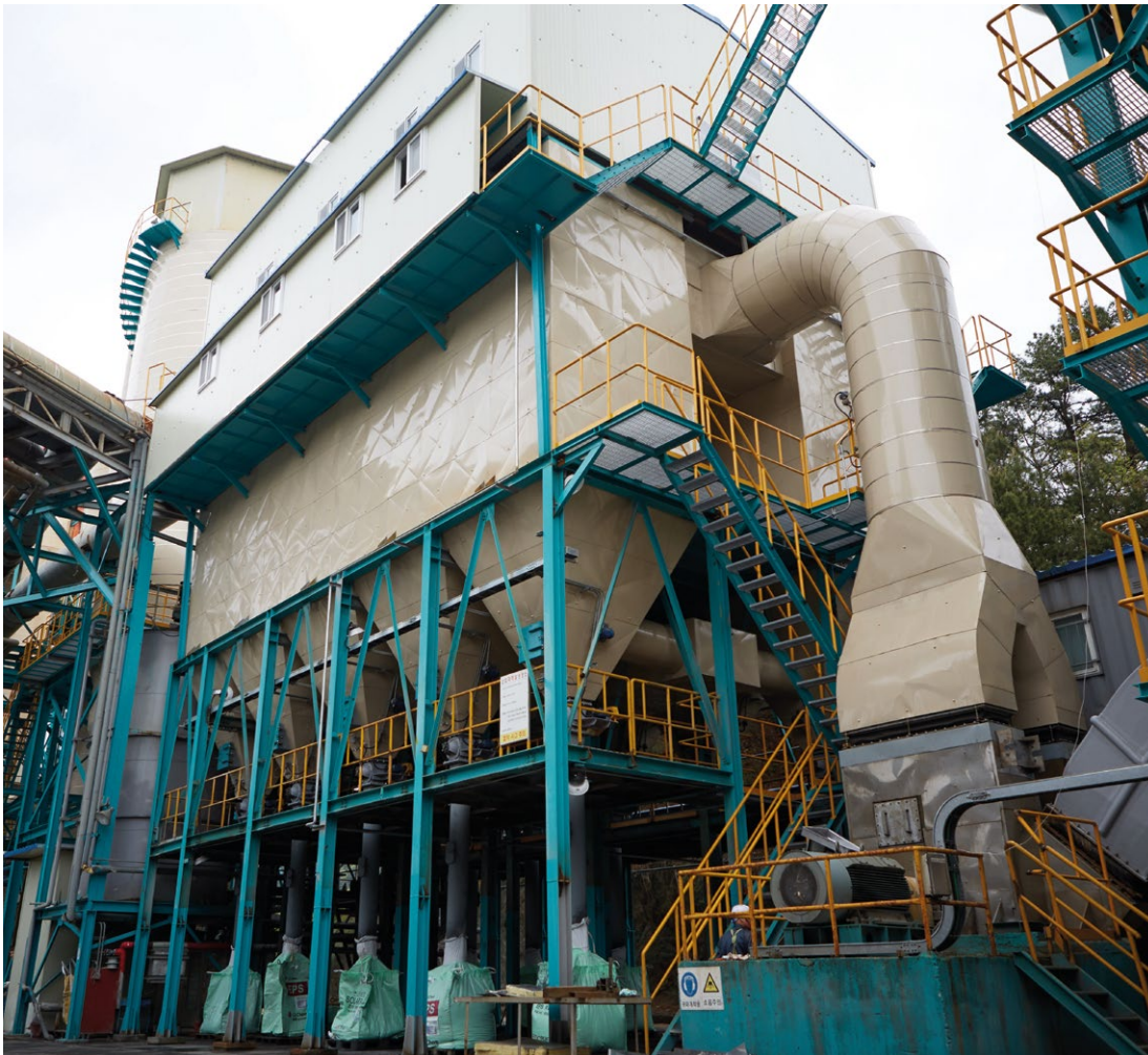
EMK operates six WTE plants and five sludge drying facilities and has the third largest incineration capacity in South Korea.
