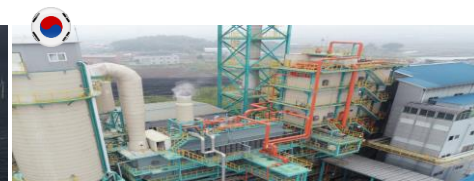
EMKH – Integrated Waste Platform 1
