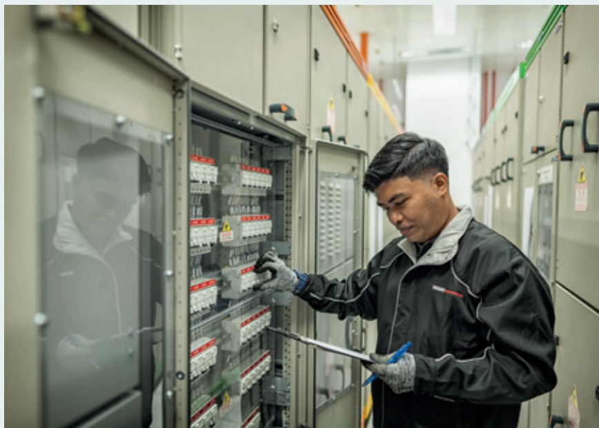
The scope of the Report covers Keppel DC REIT's colocation data centre assets, which the Manager has operational oversight of.
