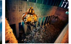
Keppel Seghers Tuas WTE Plant
