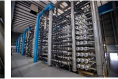
SingSpring Desalination Plant
