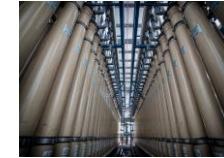
Keppel Seghers Ulu Pandan NEWater Plant
