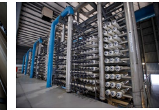
SingSpring Desalination Plant
