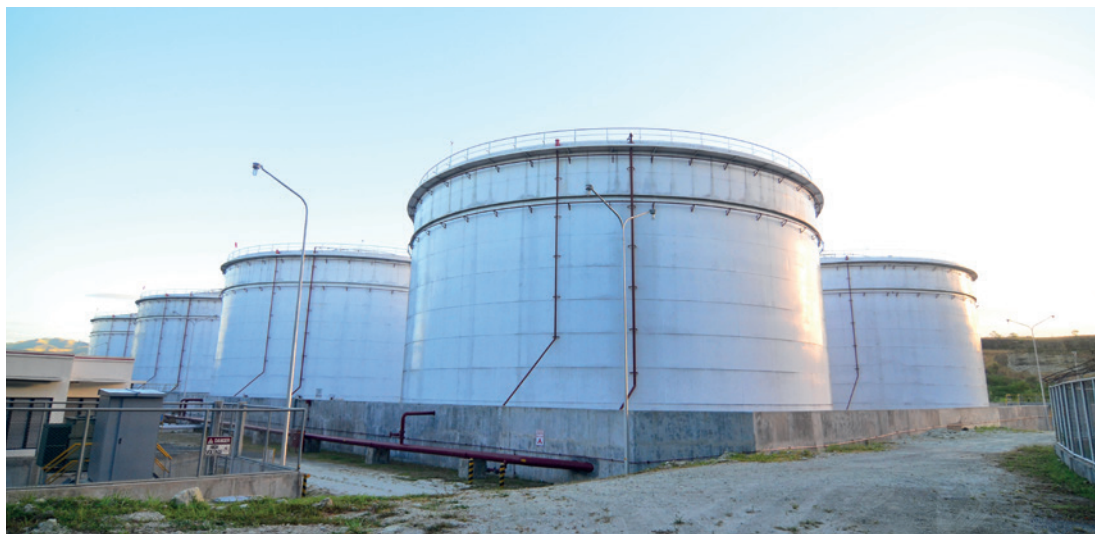
Philippine Coastal is the largest independent petroleum products storage facility in the Philippines. With the completion of tank storage expansion, capacity will increase to 6.4 million barrels.
